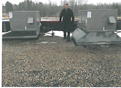
Rayco owner, Duane Nelson, walks the Burger King in Ham Lake roof to assist him in plan development.
